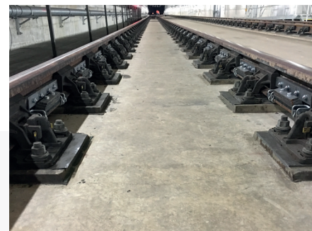
Tuned Dampers on ballastless track
