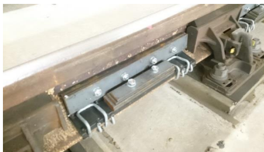
Figure 1 Installed rail damper, Perth Tunnel 6, 30 August 2016.
